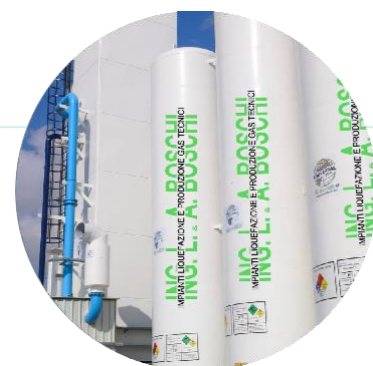
Commissioned liquid nitrogen production facility
